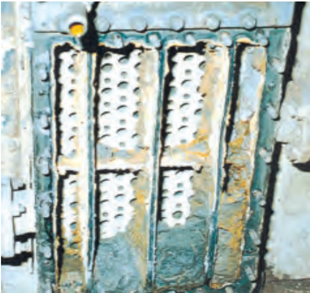
Fig. 12 — Heat exchanger after one year of service.
