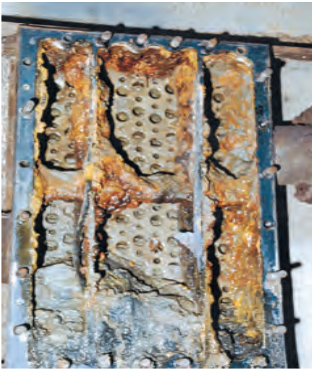
Fig. 11 — Heat exchanger before installation of magnetic water conditioner.
