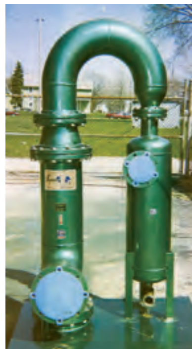
Fig. 9 — Magnetic water conditioning installation.
