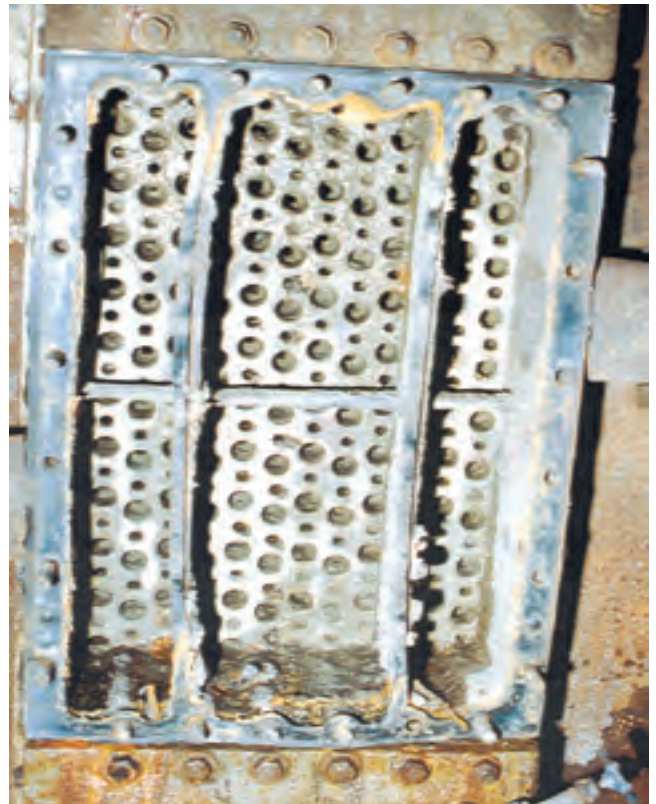
Fig. 13 — Heat exchanger washed with water hose after one year of service.
